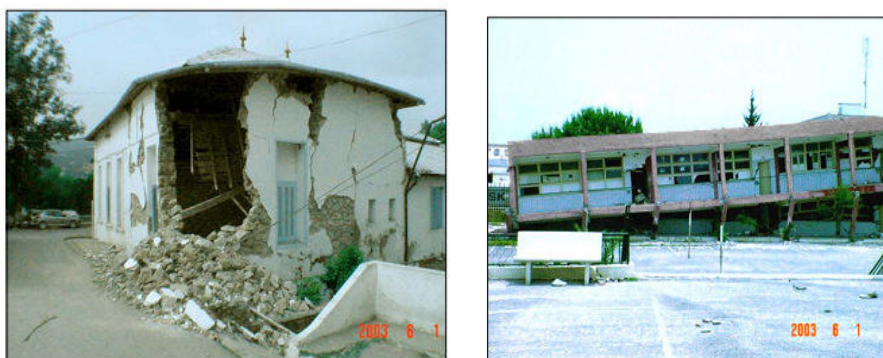
Figure4, 5***** : Damage in schools and Tenia hospital
