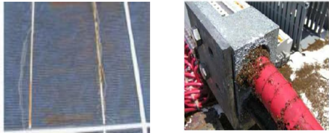
Figure 5. Examples of degradation with the impact of the climatic conditions on the photovoltaic module [6].
