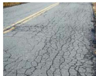
Figure 2. Fissures en carrelage.
