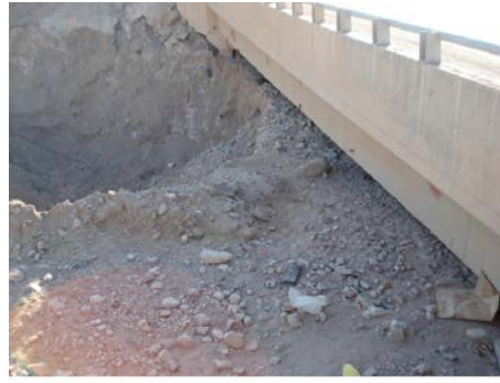
Fig. 19. Bridge after the flood
