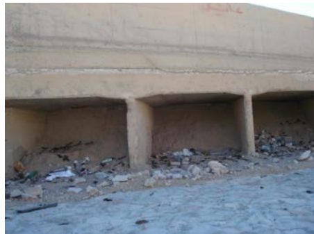
Fig. 17. Culvert after the flood
