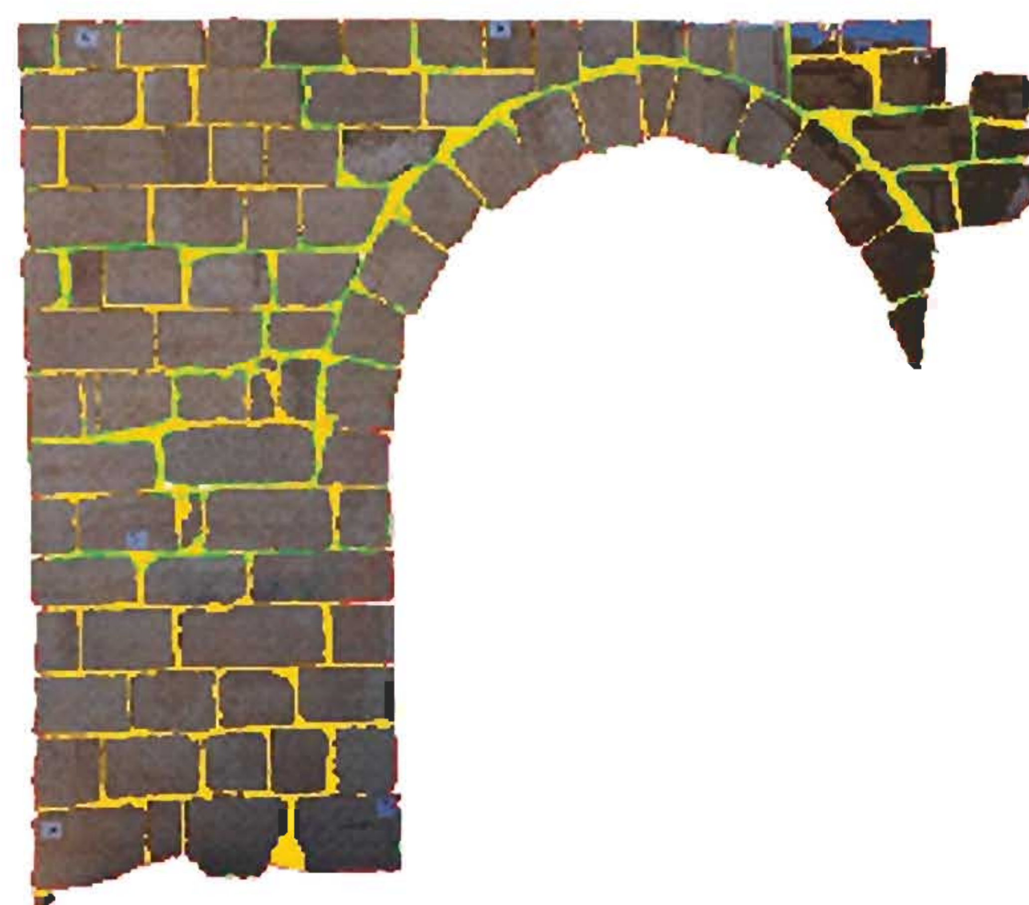
Fig. 12 Orthophoto generation on a query related to blocs, with design of USM perimeter and the cement paint in yellow
