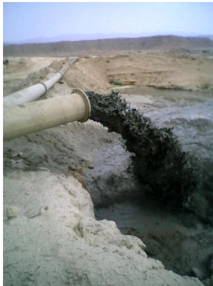
a) Draping operation carried out on the reservoir of the dam of Foug El Gherza in 2006 (Photo. Remini, 2006)
