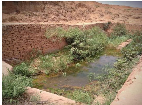
Figure 7. Tafssast Spring before rehabilitation works (Derdour, 2021)
