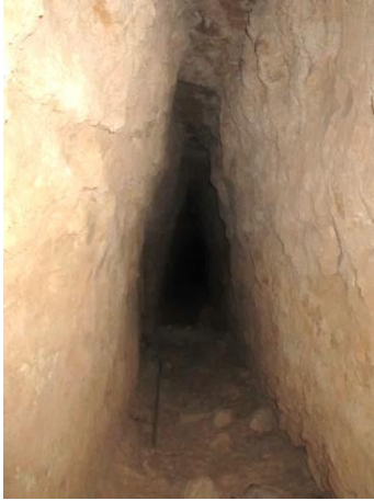
Figure 12: A triangular gallery draining the floodwaters of the Bouchemdjane seguia towards the sharing network (photo. Remini, 2014)
