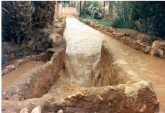
Figure 24: Collapse of garden walls under the action of water (Photo. Patrimoine de M'zab)
